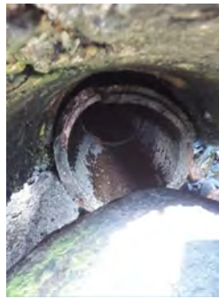
Broken Last Section of Pipe
