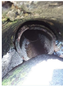
Broken Last Section of Pipe
