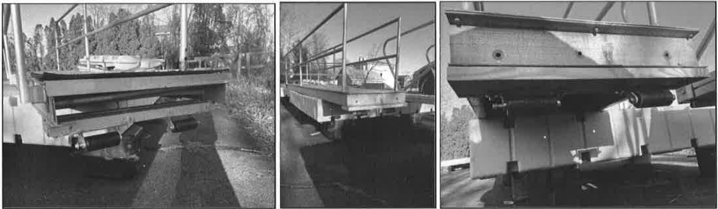
The Crew (Will, Mike, Skip, Jim Allen) installed new rollers on the gangways - saving hundreds of $$.
